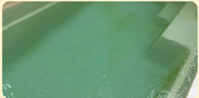
Yellow tint on the walls and steps of a plunge pool
